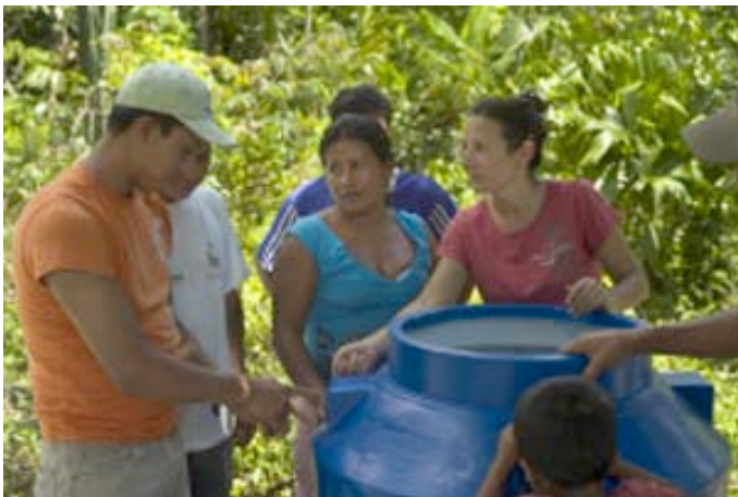
Mary helping people in the community of Isla Appai install a water system. Photograph: David Barnes
